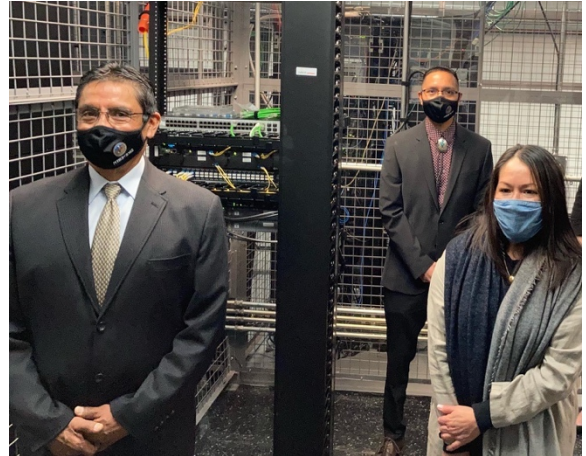
Pueblo of Jemez Governor Michael Toledo Jr. and IAD Secretary Lynn Trujillo tour a data center connecting the new Jemez broadband network to the internet.
